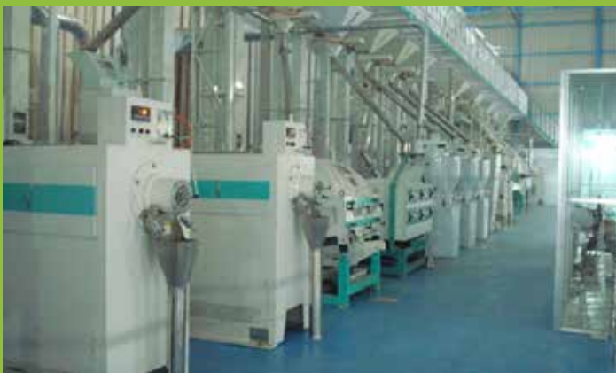
RICE MILL PLANT 100T PER DAY
