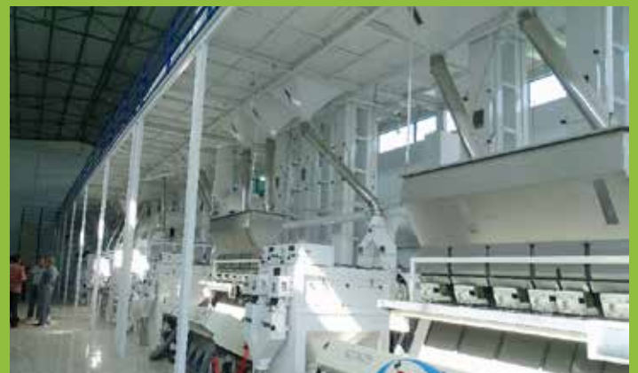
RICE MILL PLANT 150T PER DAY
